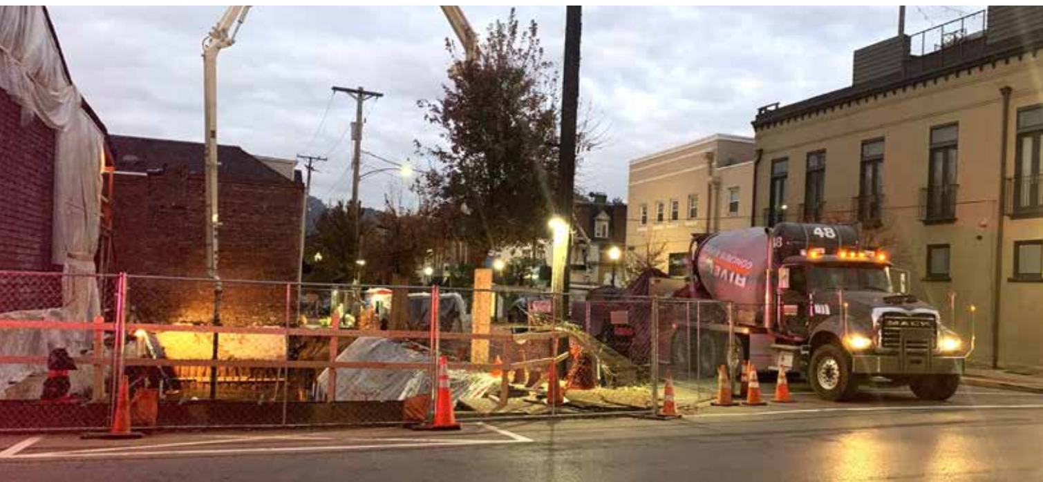
The extremely restrictive site conditions required that many of the pours and lifts be done after daytime business hours. Photo by Massaro Corporation.
